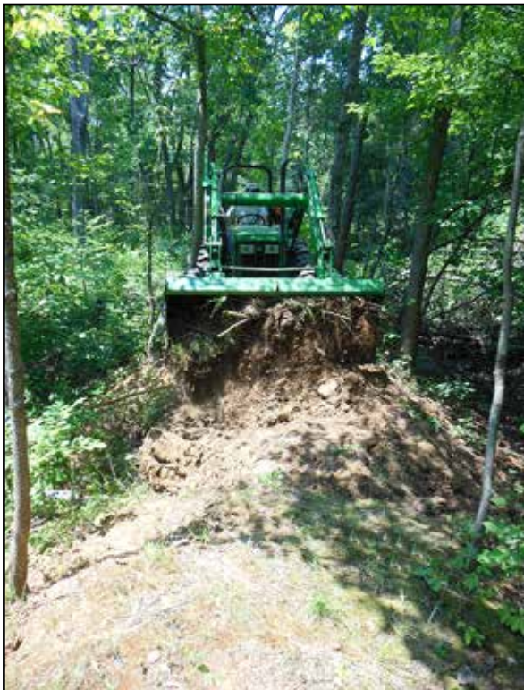
Keith Dunlap on the tractor, straddling trees to repair the dam breach to restore the western wildlife pond at the Shawnee Karst Preserve.
