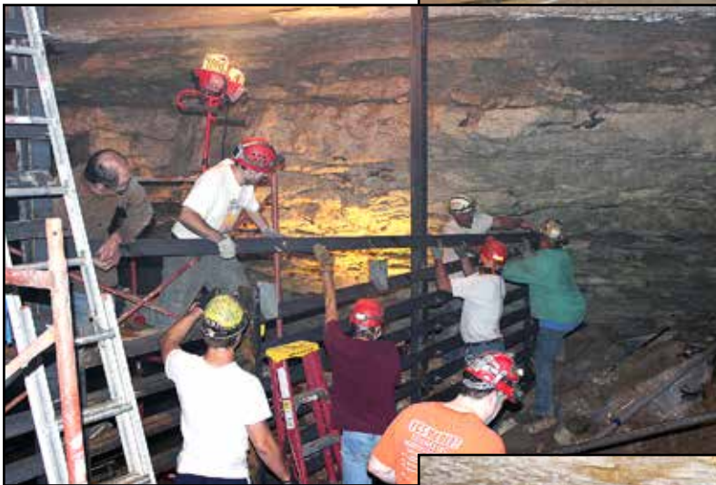
Construction of the Wyandotte Cave gate – installing the pre-fabricated door assembly (top); volunteers setting one of the horizontal bars (left); priming the finished gate (below).
