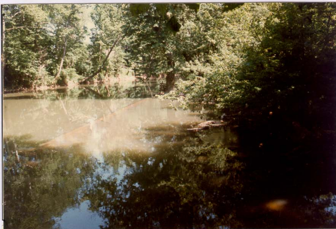
A low concrete dam (just below the water surface) constructed parallel to Indian Creek to prevent water from entering large sinks in the south bank of the creek (photo point 2).
