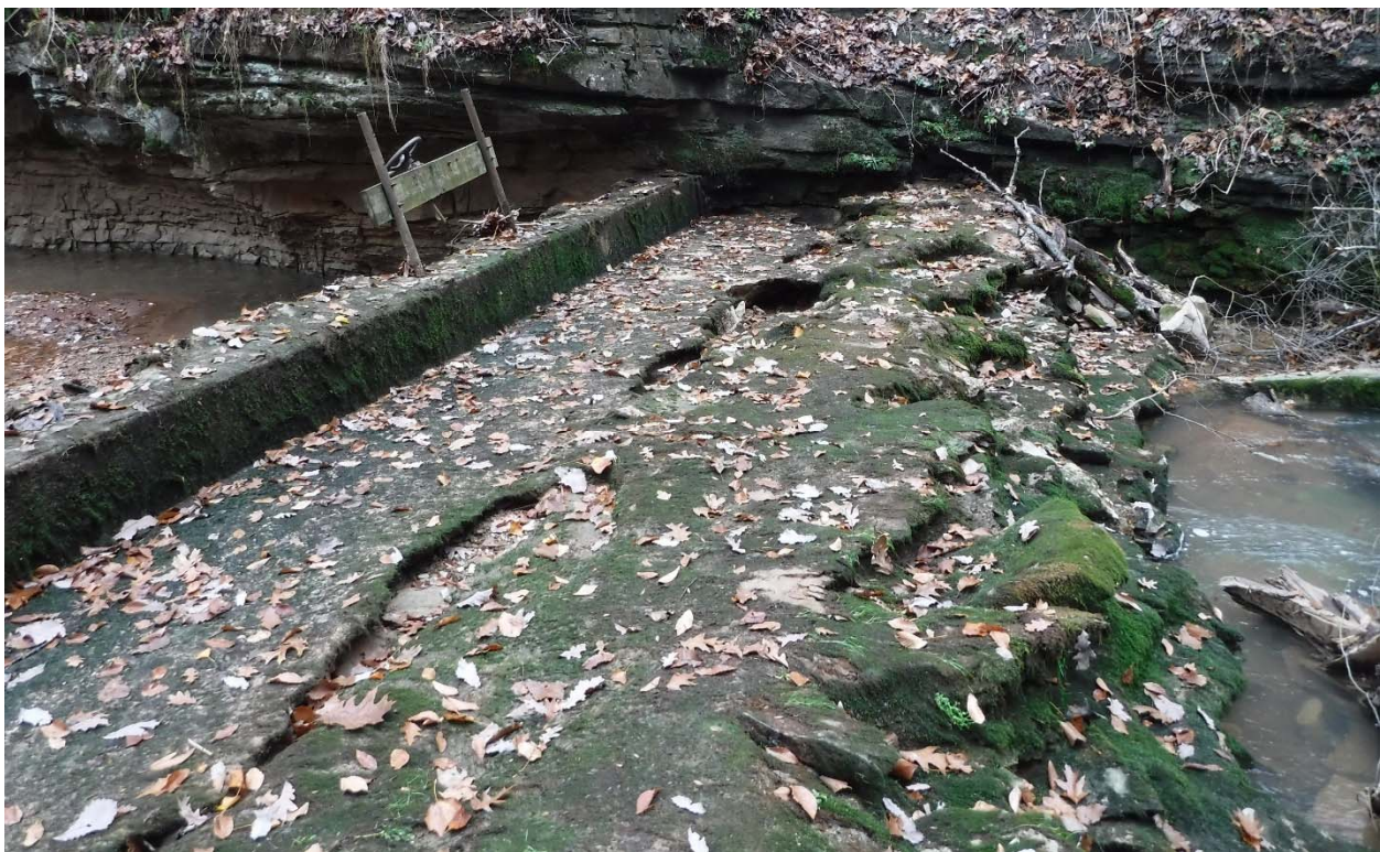
Figure 4. Dam in Upper Twin karst window in 2017. The 1937 natural stone dam is to the right, and the 1984 concrete dam is to the left. Dam is in the “open” or free-flowing position. The drainpipe runs under the center of the dams.
