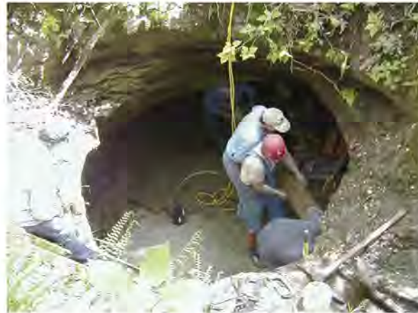
Looking down into the "pit". Gate #1 is under the ledge in the background. Steve Weinzapfel and Bruce Trotter handling steel for gate #2.
