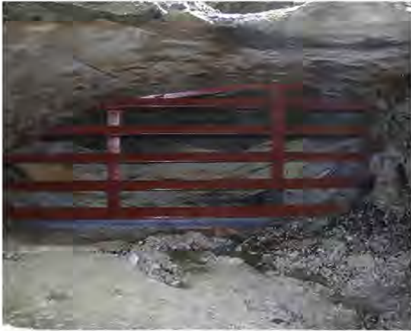
Finished gate #2 (primed but not painted). For scale, the gate is approximately ten foot wide.
