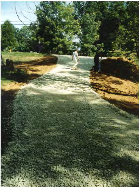
View of new driveway looking north (towards SR 54) during construction. Two culverts were installed under the driveway for drainage.
