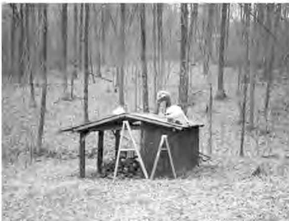
Volunteers working during Under Earth Day to re-nail the shed roof, then prime the roof and sides.
