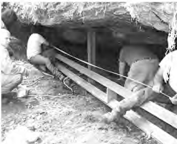
Measuring for the next horizontal bar during construction of the bat gate at Turkey Run State Park.
