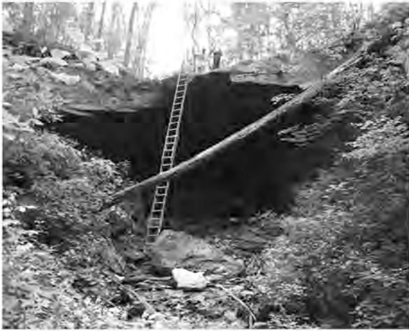
The Greene County worksite was at the base of this large sandstone shelter. All materials had to be lowered by rope or carried down the ladder.
