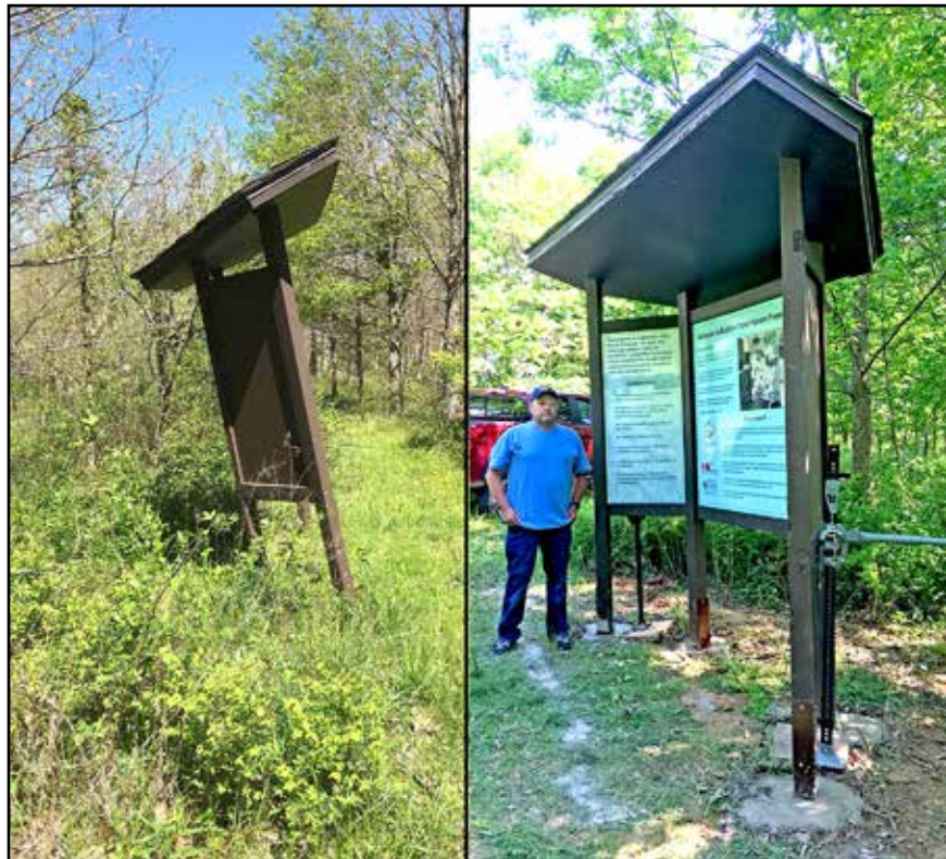
Left photo is the Buddha kiosk in early April with a significant lean due to the posts rotting off in the ground. Right photo is after the repairs on May 12th.
