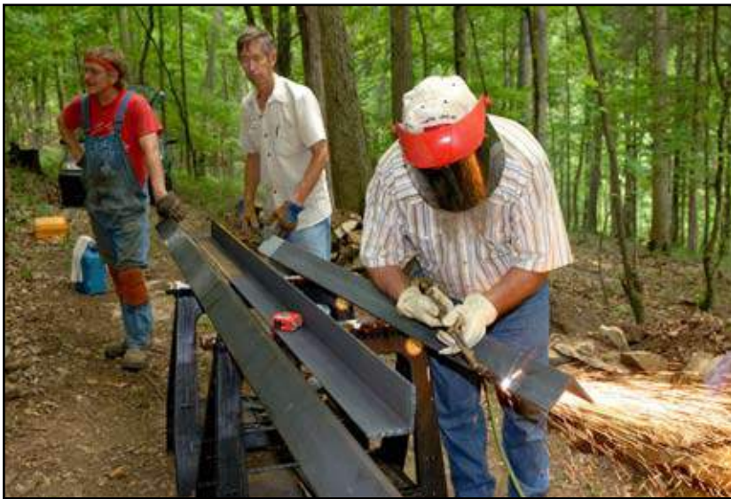
Terry Clark (foreground) is cutting the steel to the proper length while Bob Sergesketter (center) and Bruce Trotter wait to carry it into the cave.
